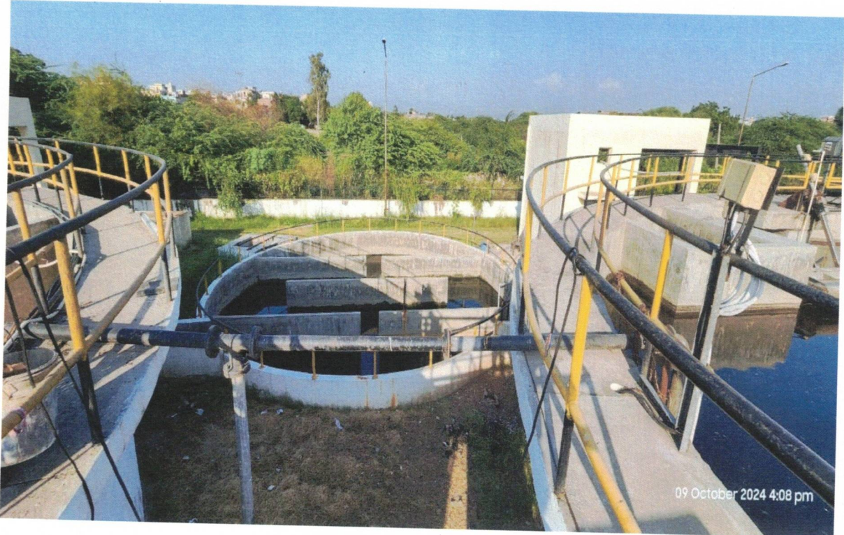
STP RAIPUR KALAN –II
